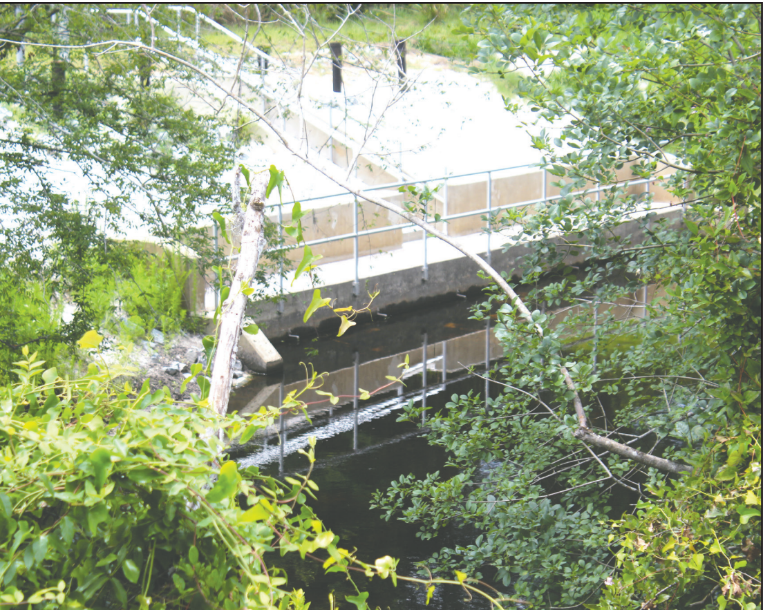
The Black Creek Water Resource Development Project's intake apparatus in the north prong of Black Creek.
